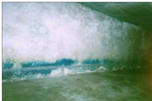
Majdanek, disinfestation wing, Room 1 with steel pipe running along wall. And blue wall staining from hydrogen cyanide exposure, particularly along the pipe. This indicates that the gas escaping from the pipe cooled down the wall drastically, making it moist, which boosted blue-pigment formation. This can be achieved with long-term use of non-toxic carbon dioxide for cooling purposes, but not with toxic carbon monoxide used during occasional short-term homicides.
